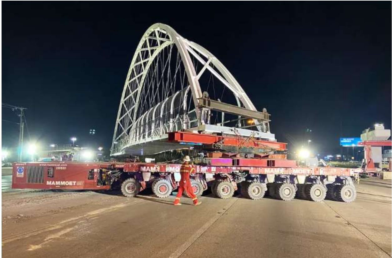
Figure 66: Construction of Northaven Trail Bridge in Dallas, Texas. Network-tied-arch constructed off-site transported and set in place (photo credit to Mike Bird and Texas Contractor).
