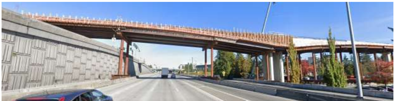
Figure 65: Falsework of Sound Transit's guideway structure on I-405 northbound traffic, looking north (photo credit to Google Map, Oct 2018).
