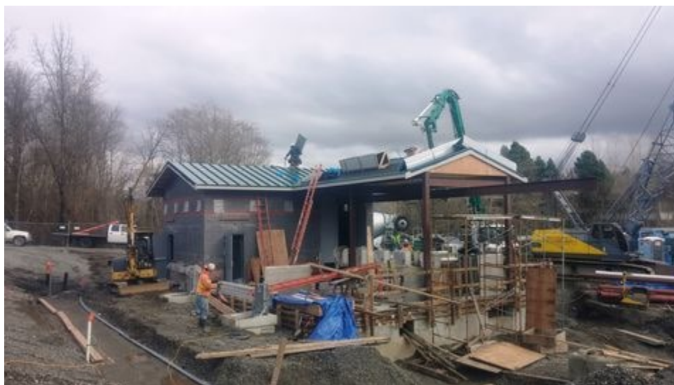
Bellefield Sewer Pump Station
