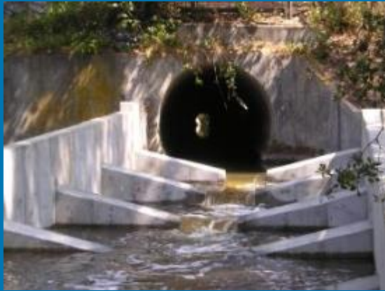
Mercer Slough Fish Ladder
