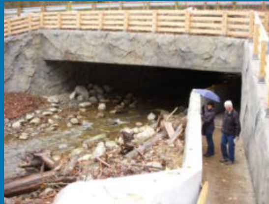
Coal Creek Parkway
