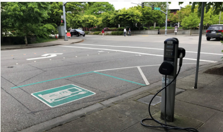
Figure 17. Bellevue On-Street EV Charger
