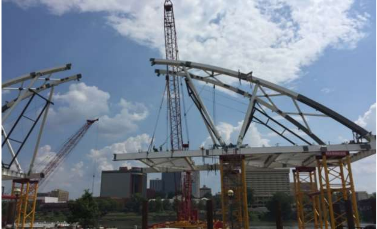
Figure 67: Construction of the Broadway Bridge in Arkansas. Segments of network-tied-arch supported by temporary support towers and temporary bracing (photo credit to Genesis Structures).
