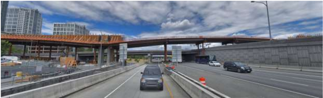
Figure 64: Falsework of Sound Transit's guideway structure on I-405 southbound traffic, looking north (photo credit to Google Map, Oct 2018).
