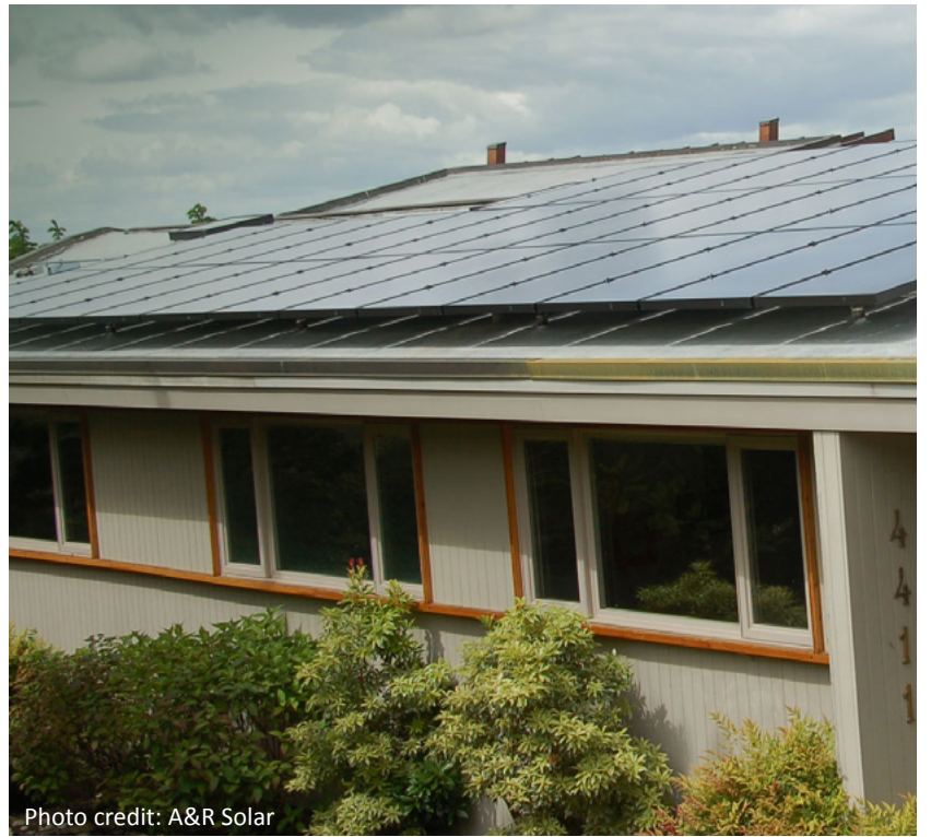
Who says the sun doesn’t shine in Bellevue? The solar array on Don and Ruth Marsh’s house cut their annual electricity bill by two-thirds.
