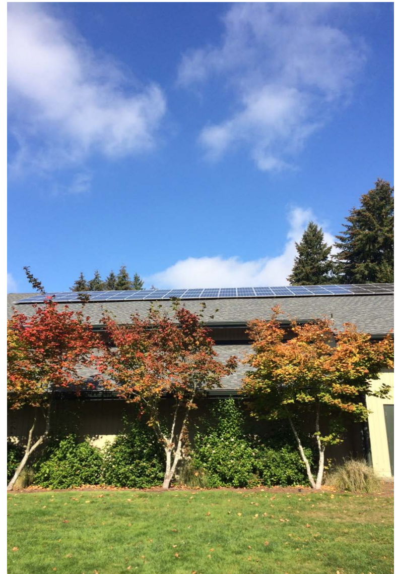
Solar array on Crossroads Community Center.
