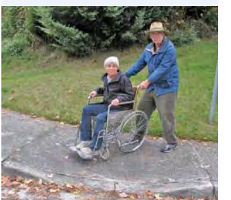
No ramp landing panel.
