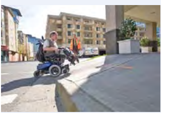
Steep ramp running slope.
